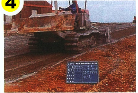
Mixing-up of the STEIN-R with the in-place soil to the bottom of the designed construction thickness
